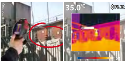
Inspecting the transformer using the Fusion Picture-in-Picture function.
