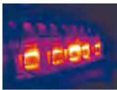
Refractory insulation defect
