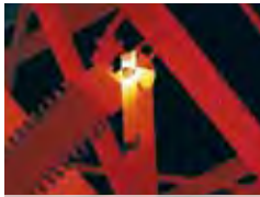
Incorrectly secured connection
