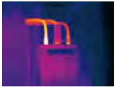
Poor connection and internal damage
